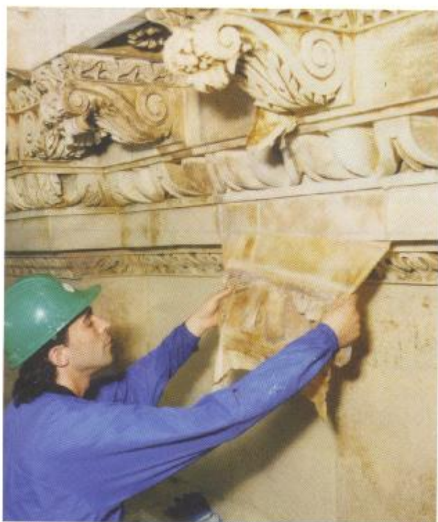
The interior stonework has been cleaned using Arte Mundit – a latex-based compound. Picture© construction photography
